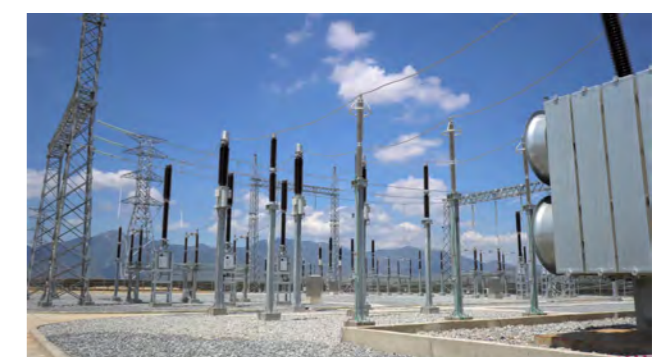
220kV Bim solar power - Ninh Thuan transmission line
