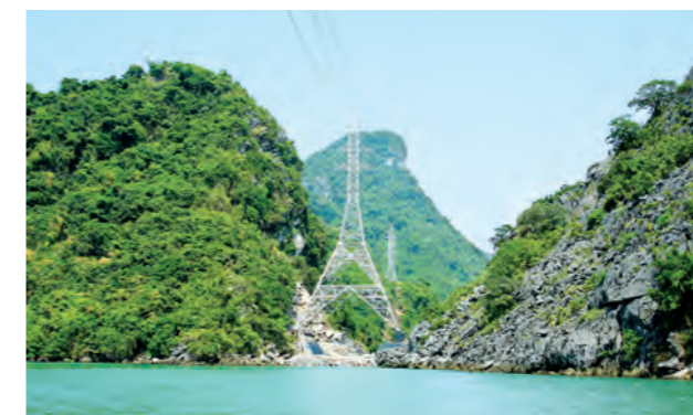
110kV transmission line bringing electricity to Co To Island district - Quang Ninh
